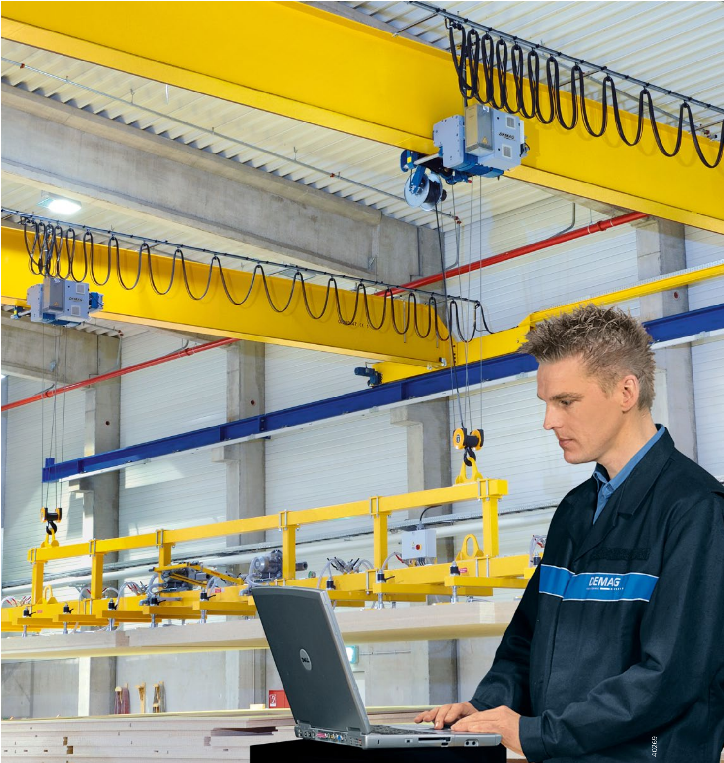
Crane system data can be read out for predictive and scheduled service.
